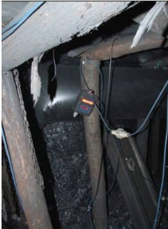
Figure 5-8: Gas Monitor Installed at Return Airway of Working Panel
